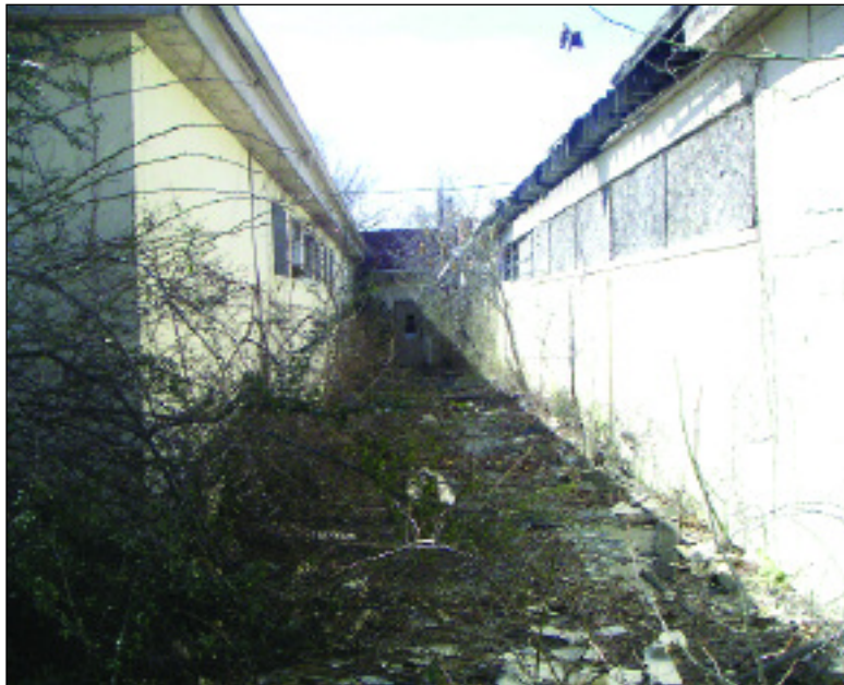
Years of neglect have left the Struthers-Dunn facilities dilapidated and potentially hazardous.
